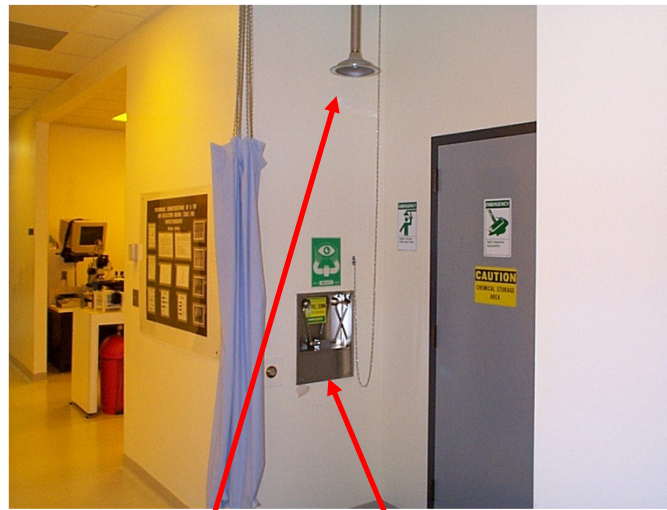
Safety shower & eyewash in between Lith Bay 1 & Lith Bay 2
