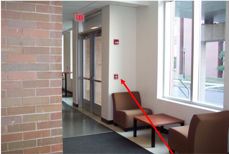
Fire alarm pull-box Outside NW Exit
